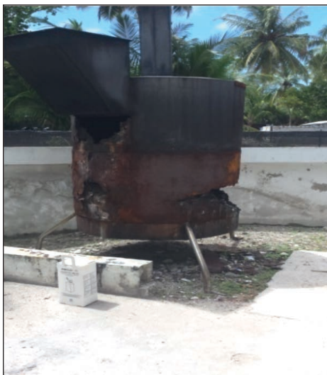
Burner in Fuvahmulah Atoll Hospital
